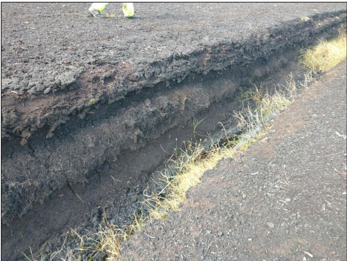
Plate 13 Drain faces obscured with collapsed and dry peat
